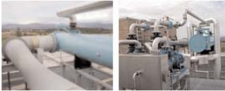
Close-up details: rooftop installation of vacuum cooling system components at Heinz' Frozen Foods plant in Dundalk, Ireland.
