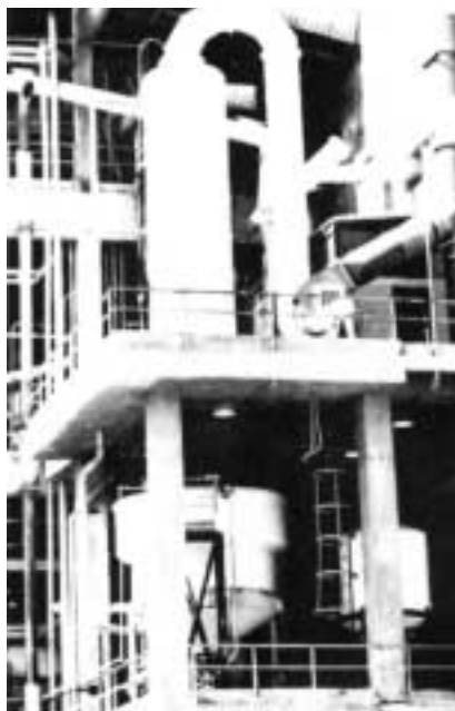
Great Northern Paper Co.'s mill in Millinocket, Maine, uses venturi scrubbers to obtain the greatest sulfur dioxide removal efficiency.
