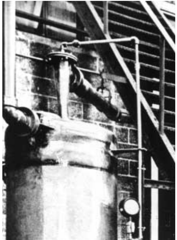
Close-up of packaged jet-venturi fume scrubber and separator at Tenneco Chemicals used for recovery of HCl Fumes during refilling or pumping operations.
