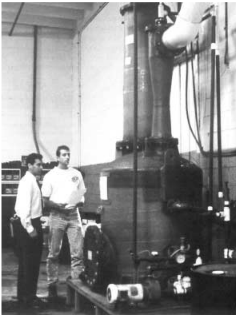
Allomatic's Paul Fathauer and Croll-Reynolds' Mark Grossman inspect the fume scrubbing system at Allomatic Products that provides more than 95% emission removal efficiency.
