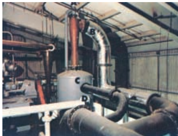
In operation, liquid hexane enters top of venturi scrubber (A), while hot vapors enter through the side (B). Vapors from separator are piped to condenser (C). 123 F preheated liquid hexane exits separator (D), and is transferred to extractor
